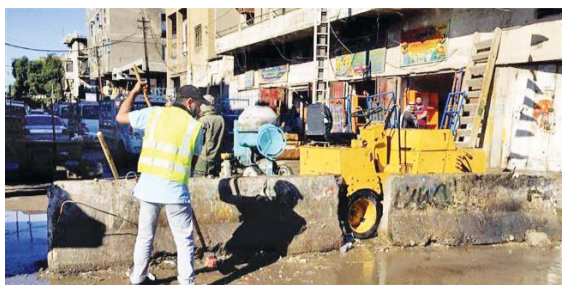
Elsewhere in al-Nasr Wal Salam city, which is also known as al-Hasuah and lies in the Abu Ghraib district of
