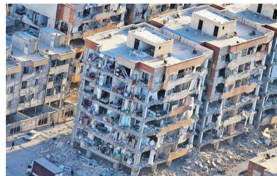
A view of buildings damaged by the magnitude 7.3 earthquake which hit western city of Sarpol-e Zahab on November 12
