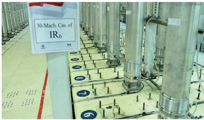
Iranian IR-6 centrifuge machines were installed in 2019 in the Natanz uranium enrichment facility near Natanz.
