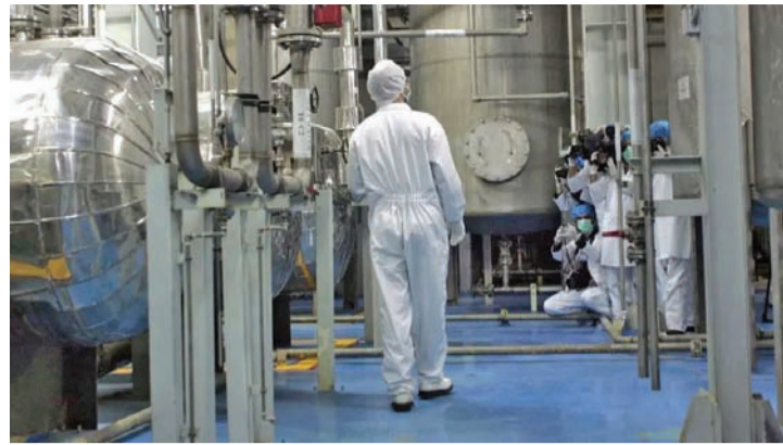
Undated photo shows one of Iran's nuclear facilities
