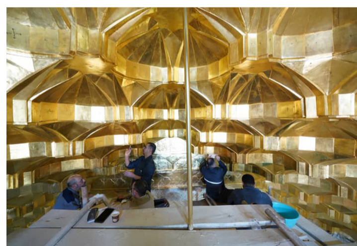
the damaged sections."
