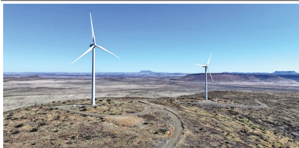
An aerial photo taken on Oct. 22, 2025 shows wind turbines of De Aar Wind Power Project in De Aar, Northern Cape, South Africa. (Xinhua/Han Xu)
